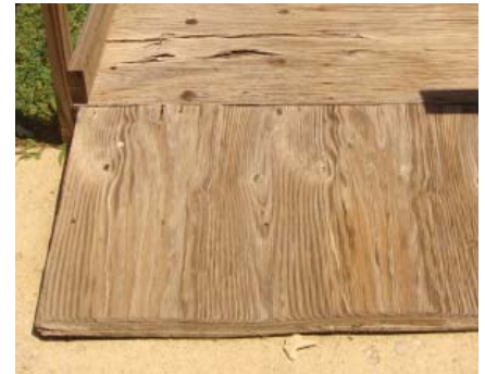
Warped and peeling surface, inch high bump to enter/exit ramp.
